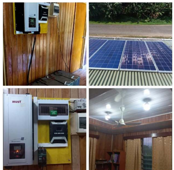
Photos of power box and solar set up.
